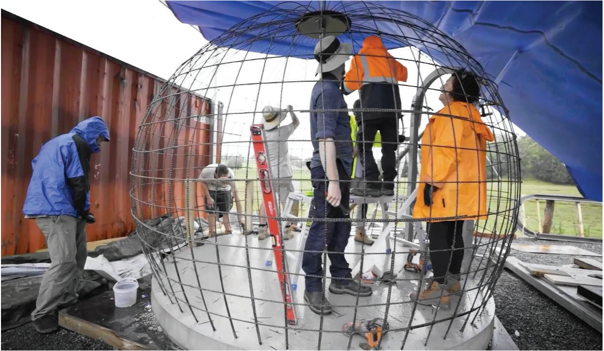
A framed up dome cage before the window and door hoods are fabricated
